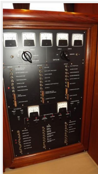
Salon Breaker Panel
