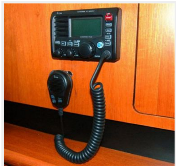
Salon VHF with Intercom to Bridge
