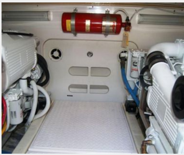
Engine Room View
