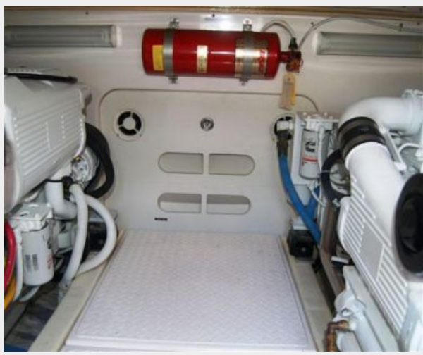
Engine Room View
