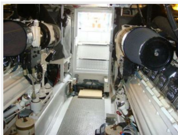
78' Buddy Davis engine room aft
