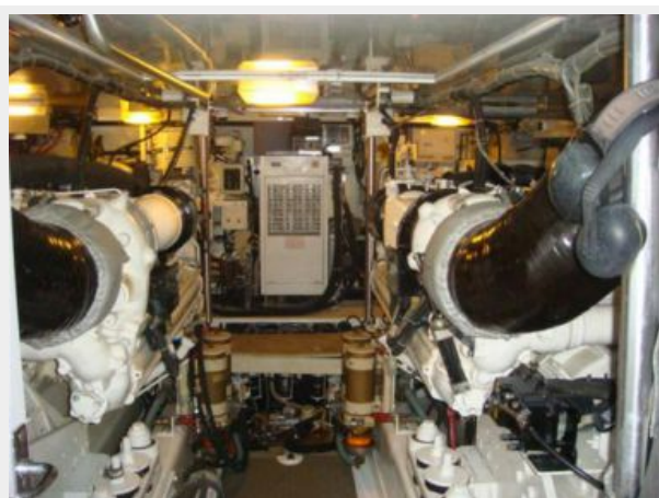
78' Buddy Davis engine room forward
