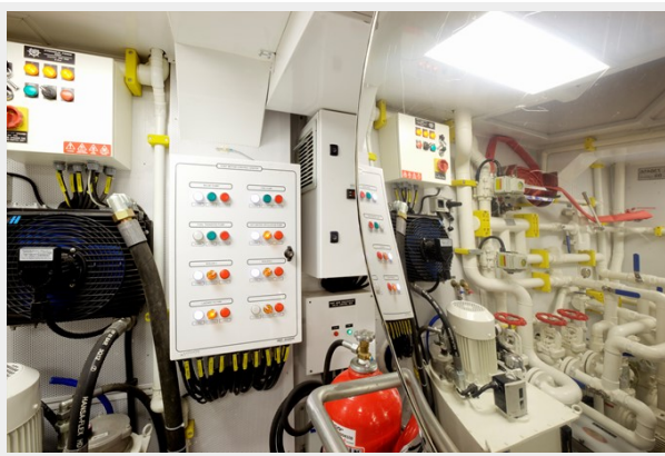
1 of 2 engine rooms
