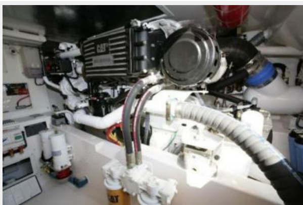
Starboard Main Engine
