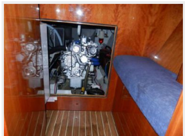
Engine Under Berth
