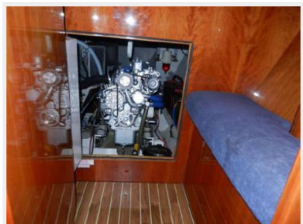
Engine Under Berth
