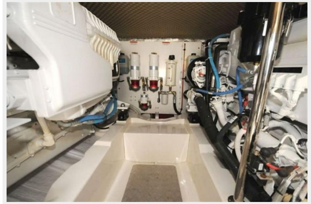
Engine Room Filters
