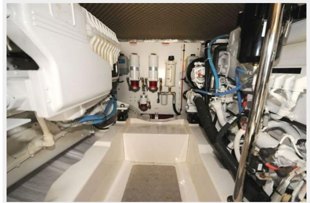
Engine Room Filters
