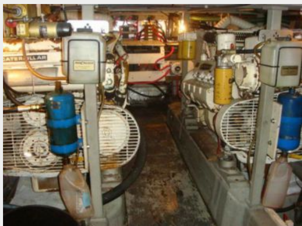
44' Tollycraft engine room aft
