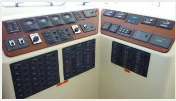
A/C & D/C Electric Monitors & Panels
