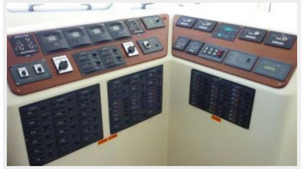
A/C & D/C Electric Monitors & Panels
