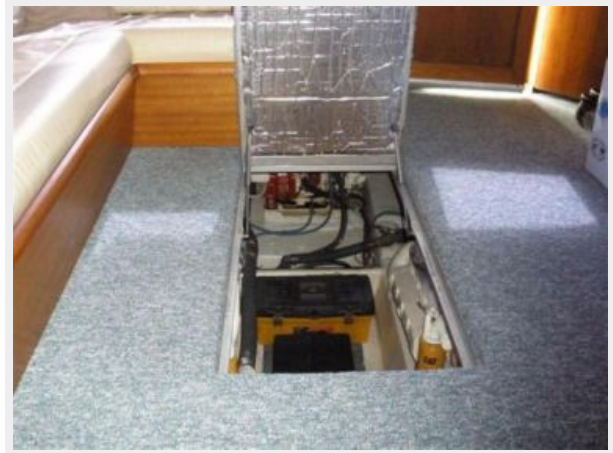
Engine Room Access
