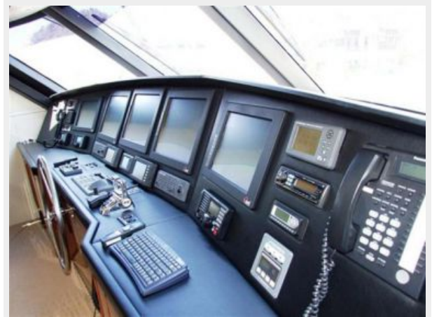
Fly Bridge Electronics
