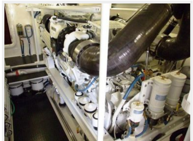
Engine Room Starboard
