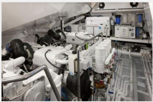
NISI Engine room
