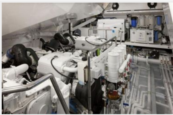
NISI Engine room
