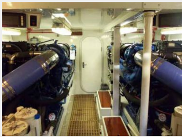
Engine Room Looking Forward
