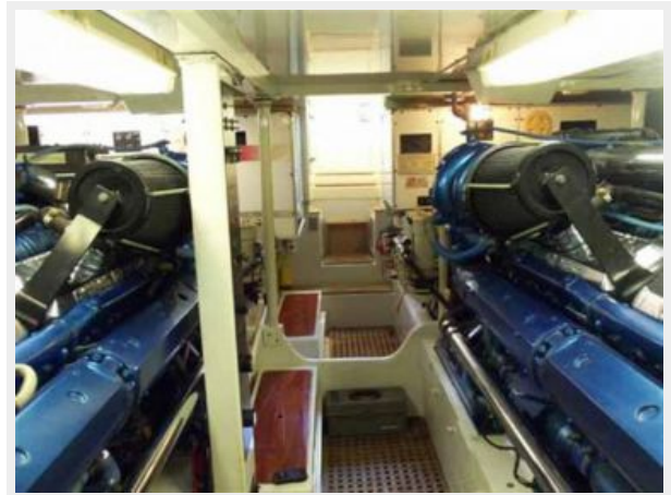
Engine Room Looking Aft
