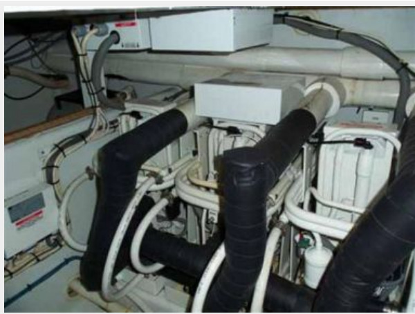
Triple Chilled Water Compressor
