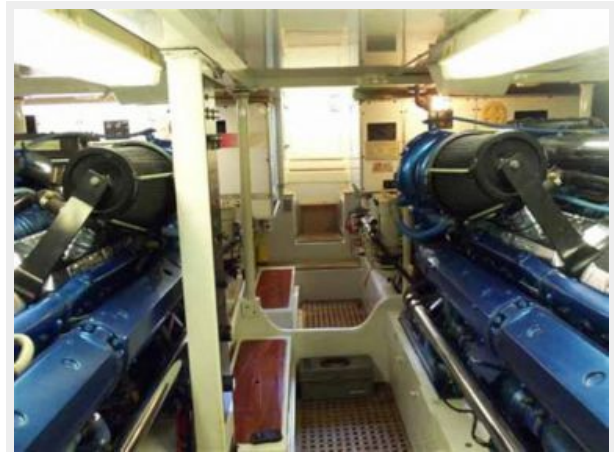
Engine Room Looking Aft
