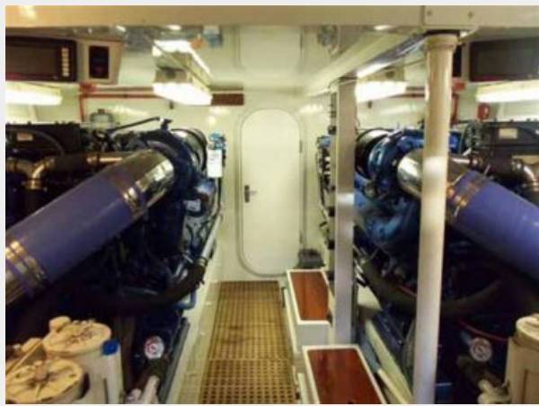
Engine Room Looking Forward
