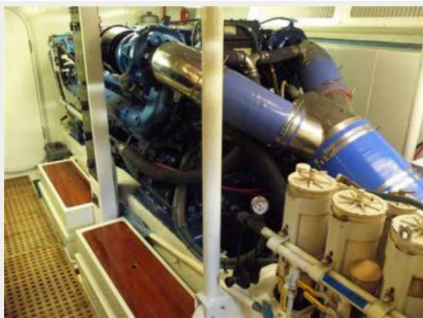
Starboard Engine Room
