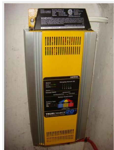
35' C&C battery charger
