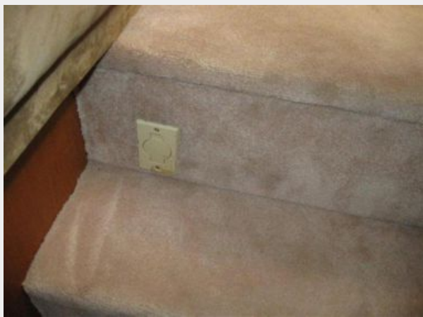
Galley 2 - Central Vacuum System
