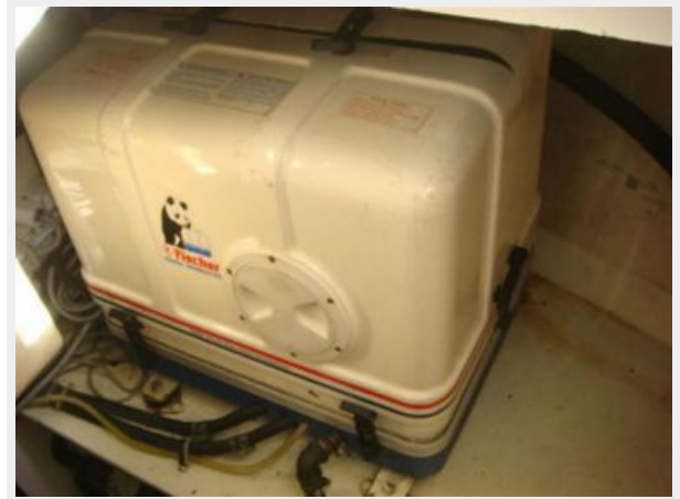
51' Little Harbor generator1
