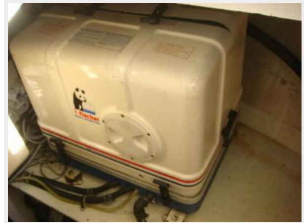
51' Little Harbor generator1
