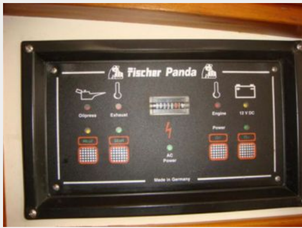
51' Little Harbor generator panel
