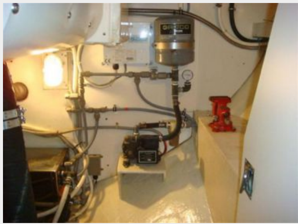
51' Little Harbor engine room aft
