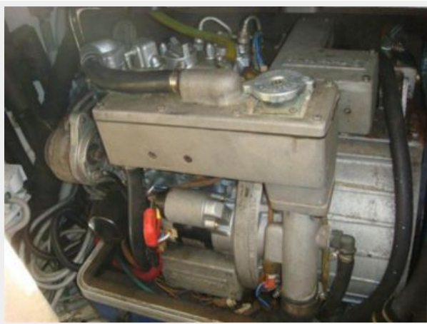
51' Little Harbor generator2
