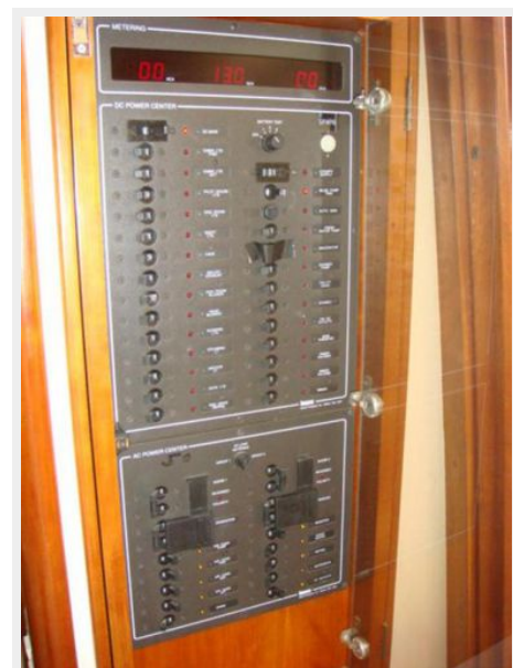
51' Little Harbor electrical panel
