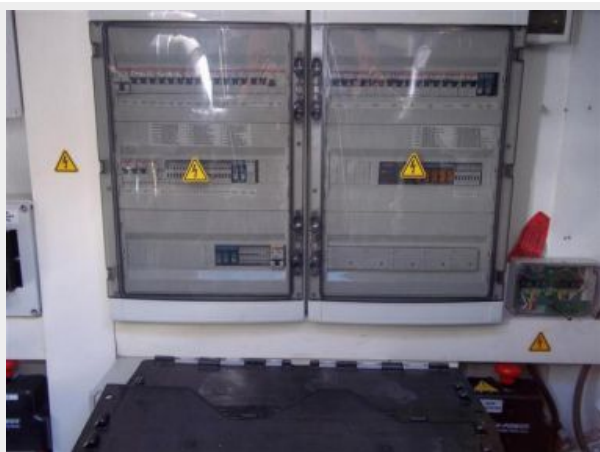
Engine Room - Electric Panel
