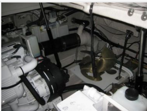
Engine Room w/ Spare Props
