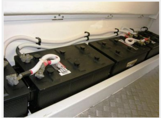
(2) 24V Battery Banks
