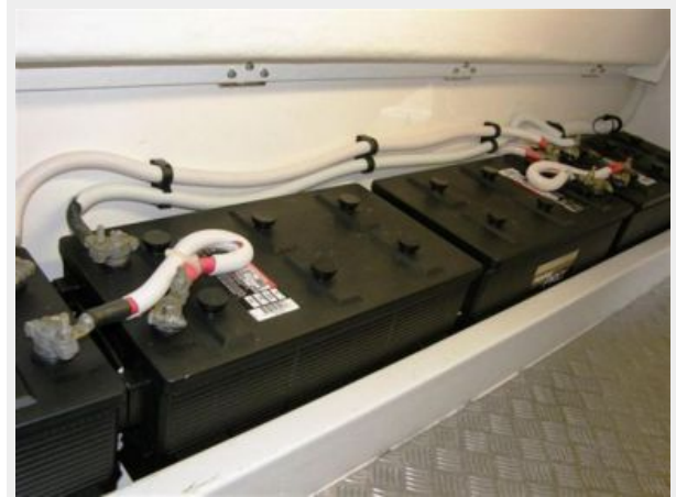
(2) 24V Battery Banks
