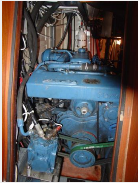
Engine Room, Forward
