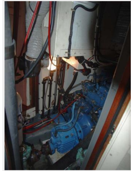
Engine Room, Aft
