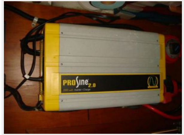
44' North Shore Trawler inverter
