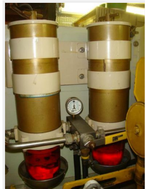
44' North Shore Trawler Racor fuel filters
