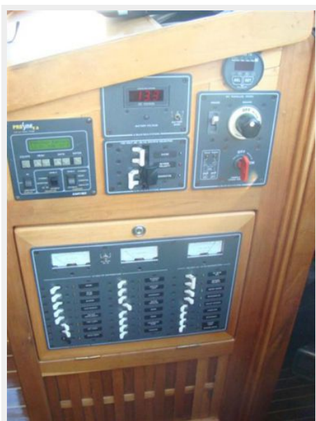
44' North Shore Trawler electrical panel
