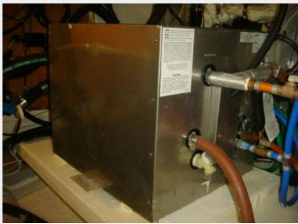
44' North Shore Trawler water heater
