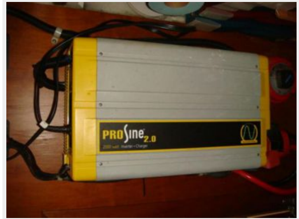
44' North Shore Trawler inverter
