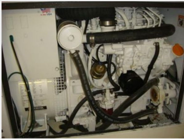
44' North Shore Trawler generator
