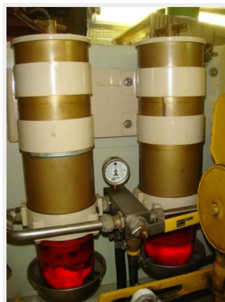
44' North Shore Trawler Racor fuel filters
