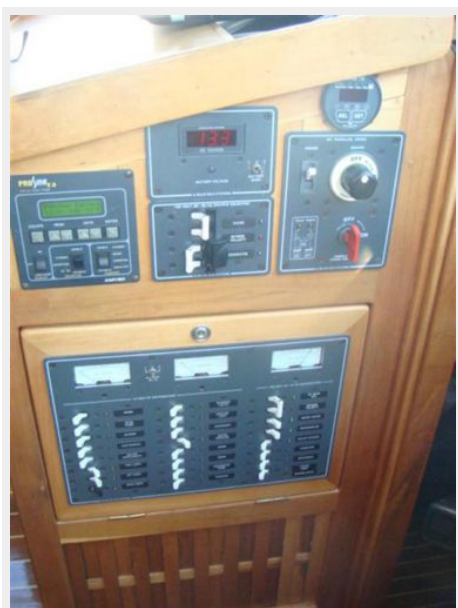
44' North Shore Trawler electrical panel
