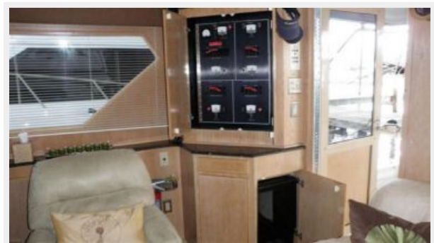
Electrical panels / Icemaker
