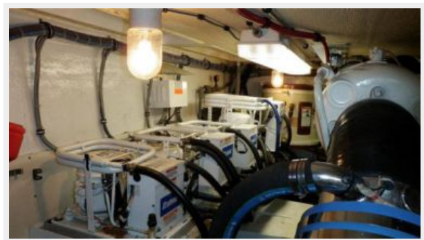
Outboard of port engine facing forward
