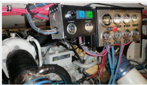
Engine Room mechanical gauges
