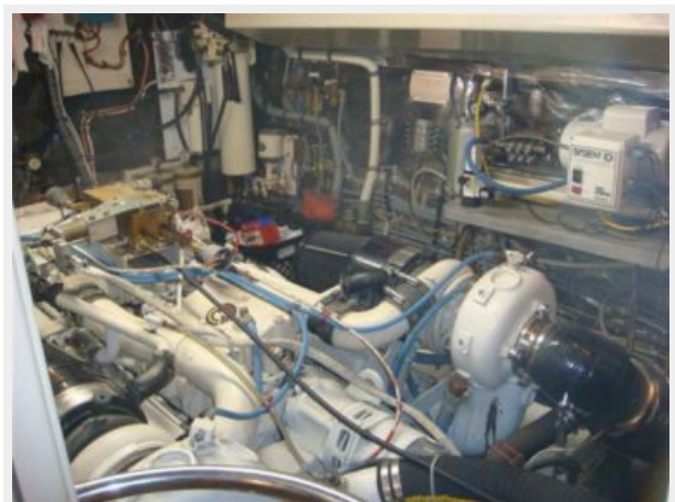
70' Hatteras Motoryacht starboard engine room
