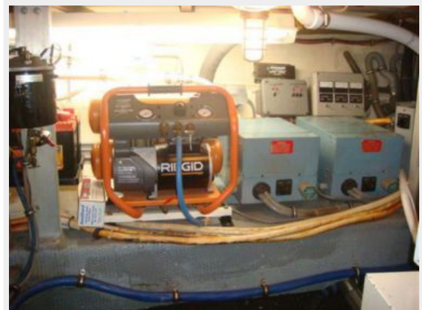
70' Hatteras Motoryacht generator room starboard
