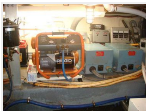
70' Hatteras Motoryacht generator room starboard
