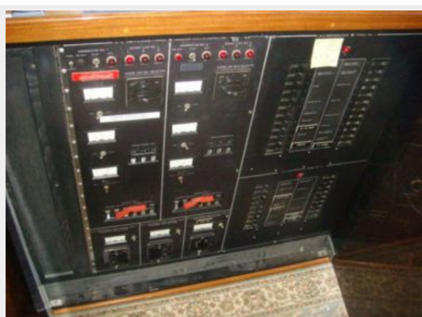
70' Hatteras Motoryacht electrical panel2
