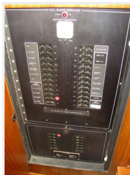
70' Hatteras Motoryacht electrical panel1
