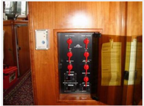
Battery Control Panel
