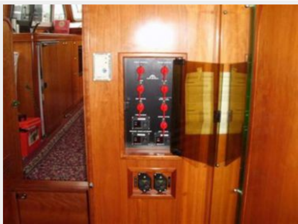
Battery Control Panel
