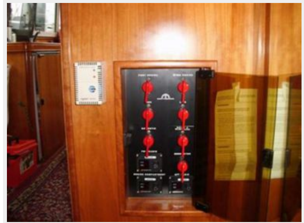
Battery Control Panel
