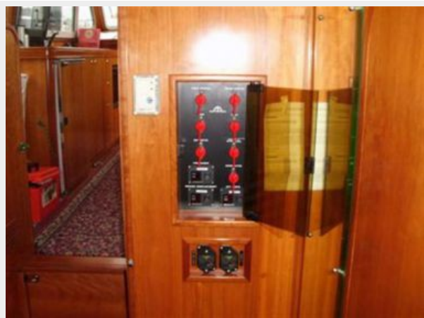
Battery Control Panel
