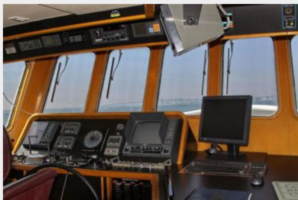
Wheel House Instrumentation
