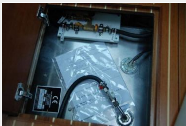
Extra Diesel Tanks
