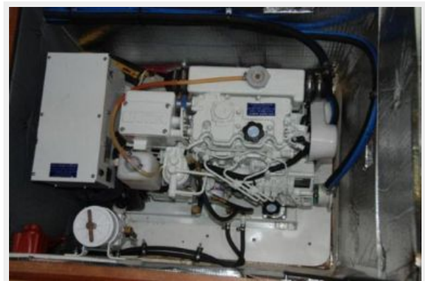
Extra Large Genset
