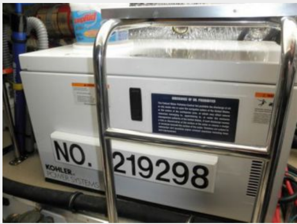
Generator in Sound Shield
