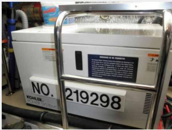
Generator in Sound Shield
