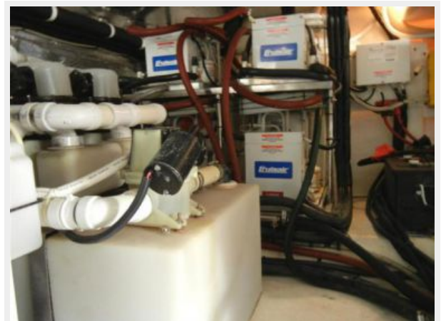
A/C units, holding tank
