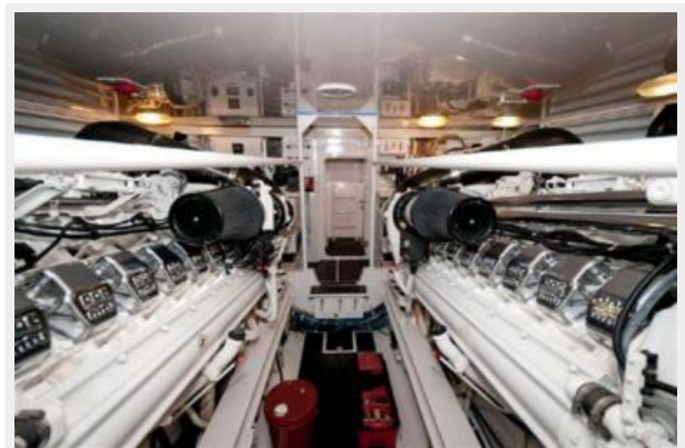
Crew Quarters access door to engine room
