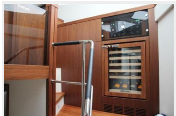
Wine Cooler and Electrical Panel
