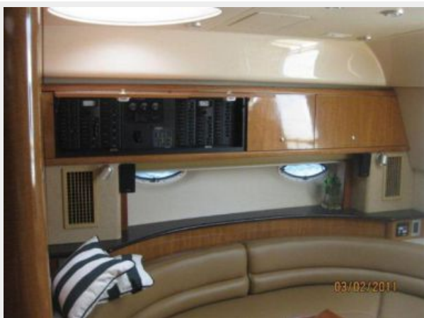
Electrical System 1 - AC / DC Panel
