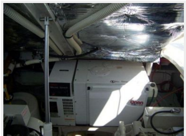
Electrical System 2 - Generator
