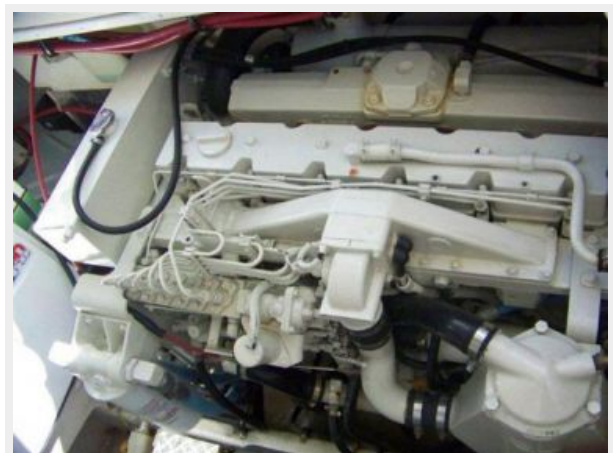
Engine and Mechanical Equipment 2
