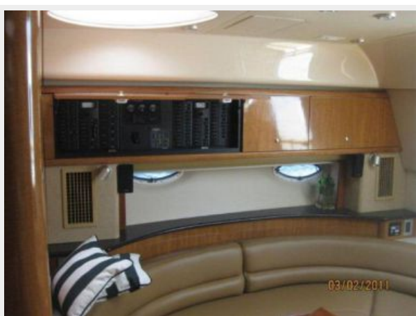
Electrical System 1 - AC / DC Panel
