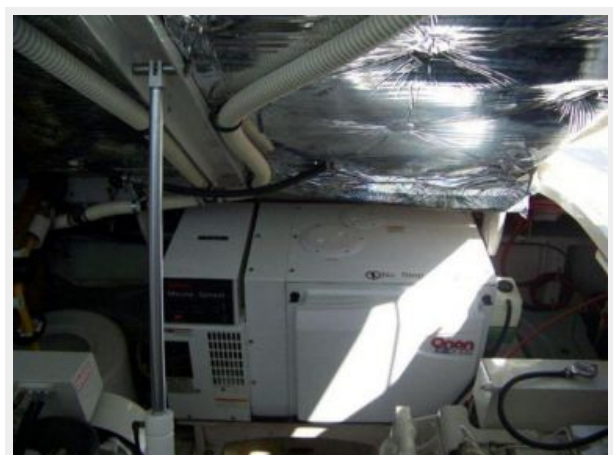
Electrical System 2 - Generator
