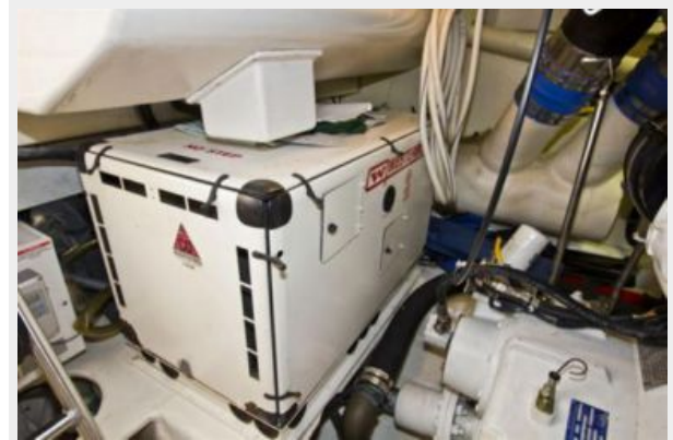
Engine Room Generator
