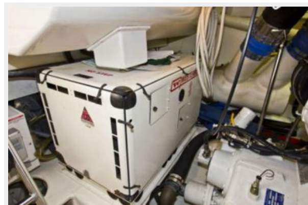
Engine Room Generator
