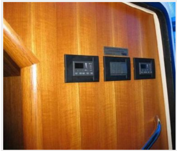
Air Conditioning Controls
