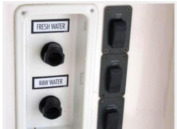
Cockpit Washdown Controls
