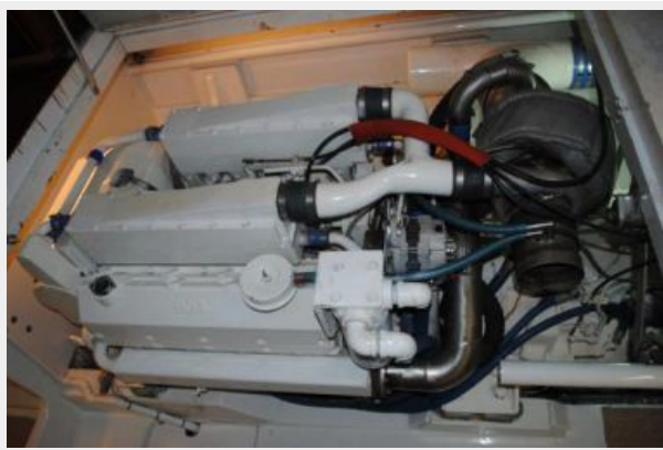
Starboard Top Engine
