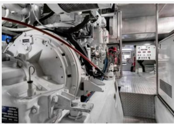
Engine Room (Note: Engine replaced w/ NEW John Deere 2013)
