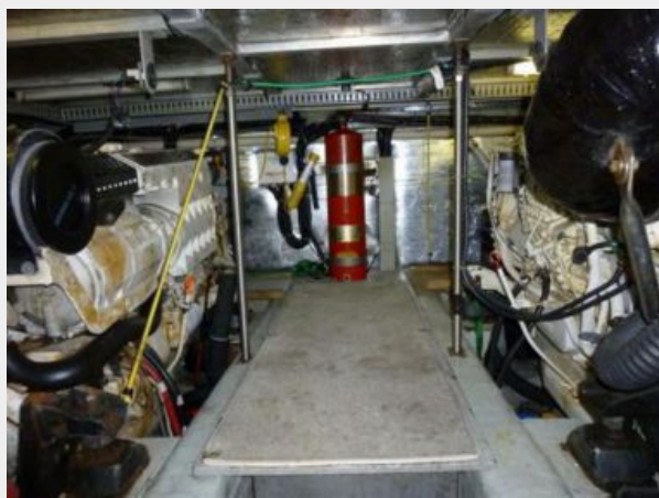
Carver 450 engine room
