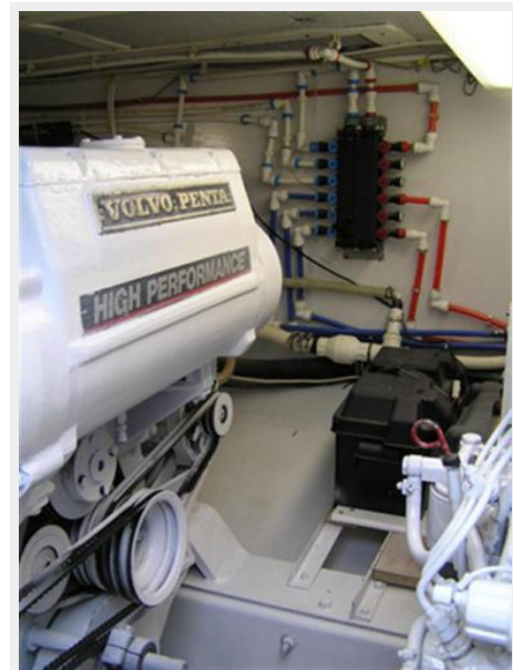
Port Engine Water
